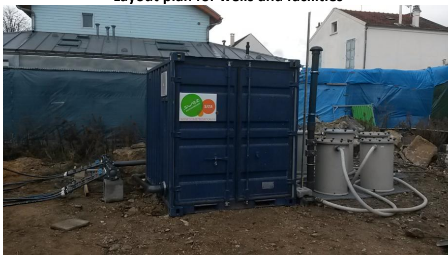
Photograph of SVE treatment facilities
